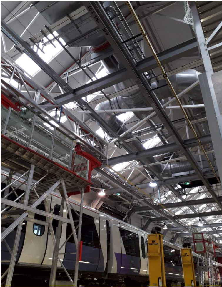
Fan shown in roof apex
