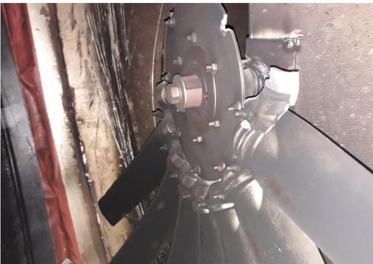
Damaged extraction unit
