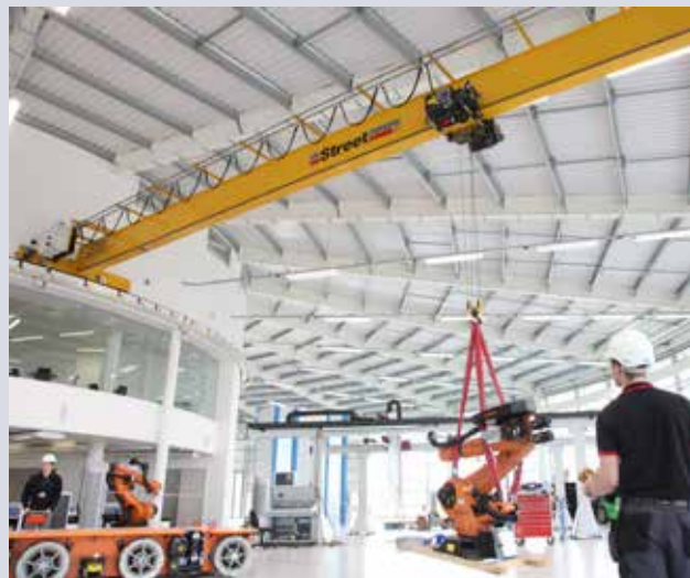
ZX cranes forms an essential part of operations in this iconic circular factory.
